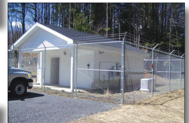
Another view of the plant with service truck
