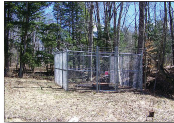
New collection well with submersible pumps
