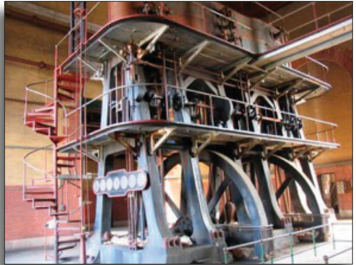
Holly steam powered pumps
